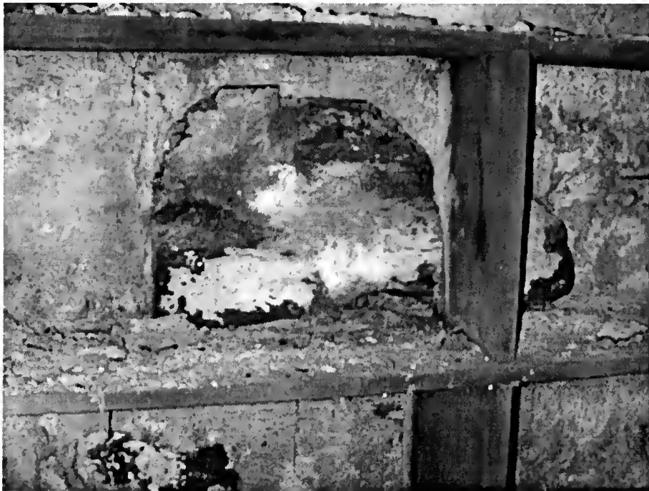
Figure 11 Stone Jutting from the Interior Masonry Wall in the Basement of the Center Section of the Main House, 2002
